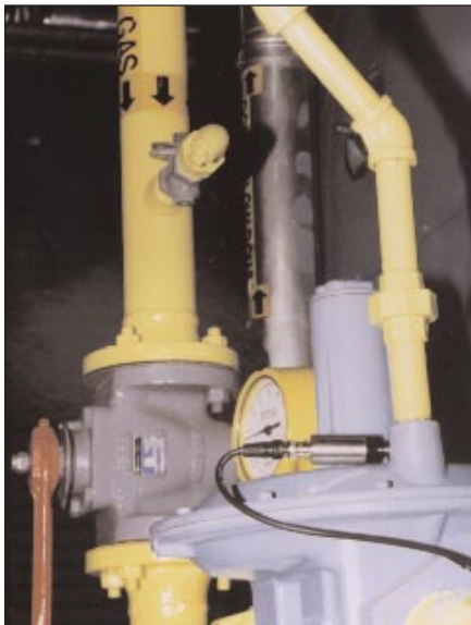
Safety valve leaks.
