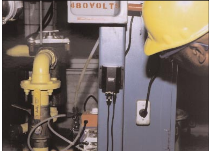
UCA has local alarm and power indicators.
